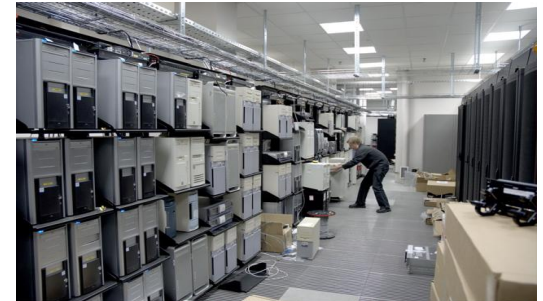
State-of-the-art, 3300 sq. ft shared engineering lab
